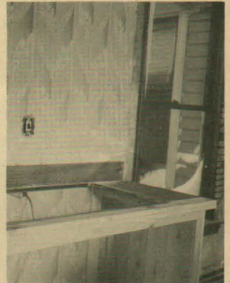
This room is being converted to a kitchen. The sink top and cabinets will be built in. All new plumbing will be provided.
